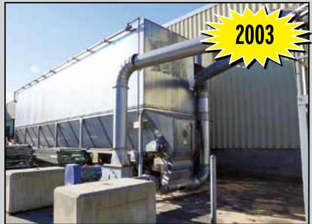
DISA DUST COLLECTION SYSTEM
