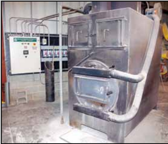
BIOMASS COMBUSTION SYSTEMS WASTE WOOD FURNACE WITH CONTROLS
