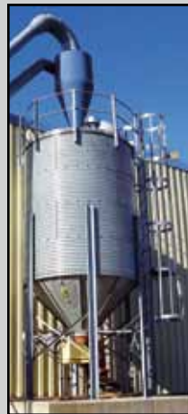
FEED SILO FOR WASTE WOOD FURNACE
