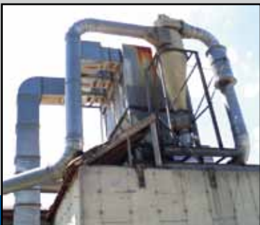
(1 OF 2) NORFAB CENTRAL DUST COLLECTION SYSTEMS
