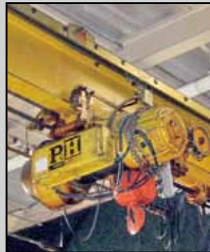
(1 OF 5) 5-TON BRIDGE CRANES
