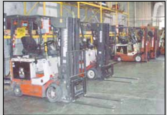
VIEW OF ELECTRIC FORKLIFTS AND CHARGERS
