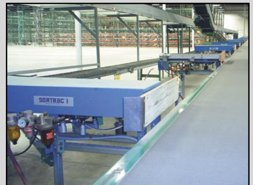
SAMPLE CONVEYOR W/SORTRAC DIVERTERS
