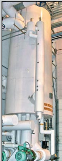
(1 OF 2) PRIMARY INSULATED AMMONIA TANKS
