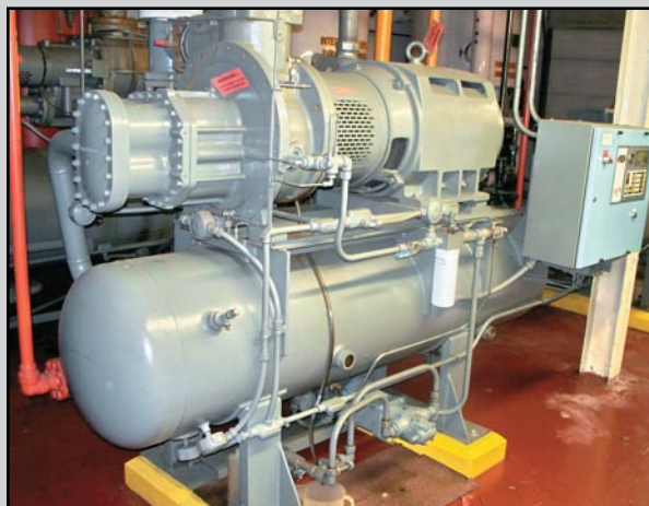
(1 OF 4) 250-400 HP AMMONIA COMPRESSORS
