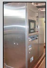
PLC CONTROLS- BAGEL SEEDING LINE
