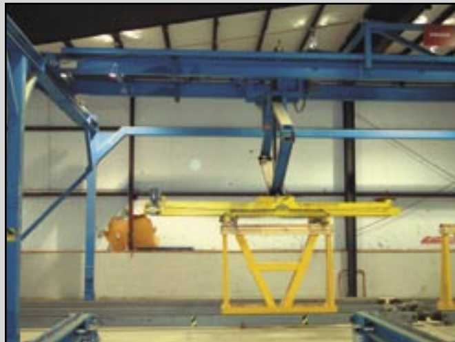
FINISHED PANEL HANDLING CRANE
