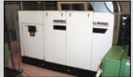
(1 OF 2) INGERSOLL-RAND AIR COMPRESSOR
