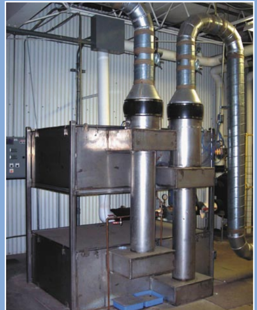
DRY BED GAS SCRUBBER SYSTEM
